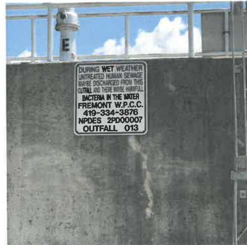
Non-pumped CSO location
